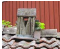
Ventilation genom taket.
